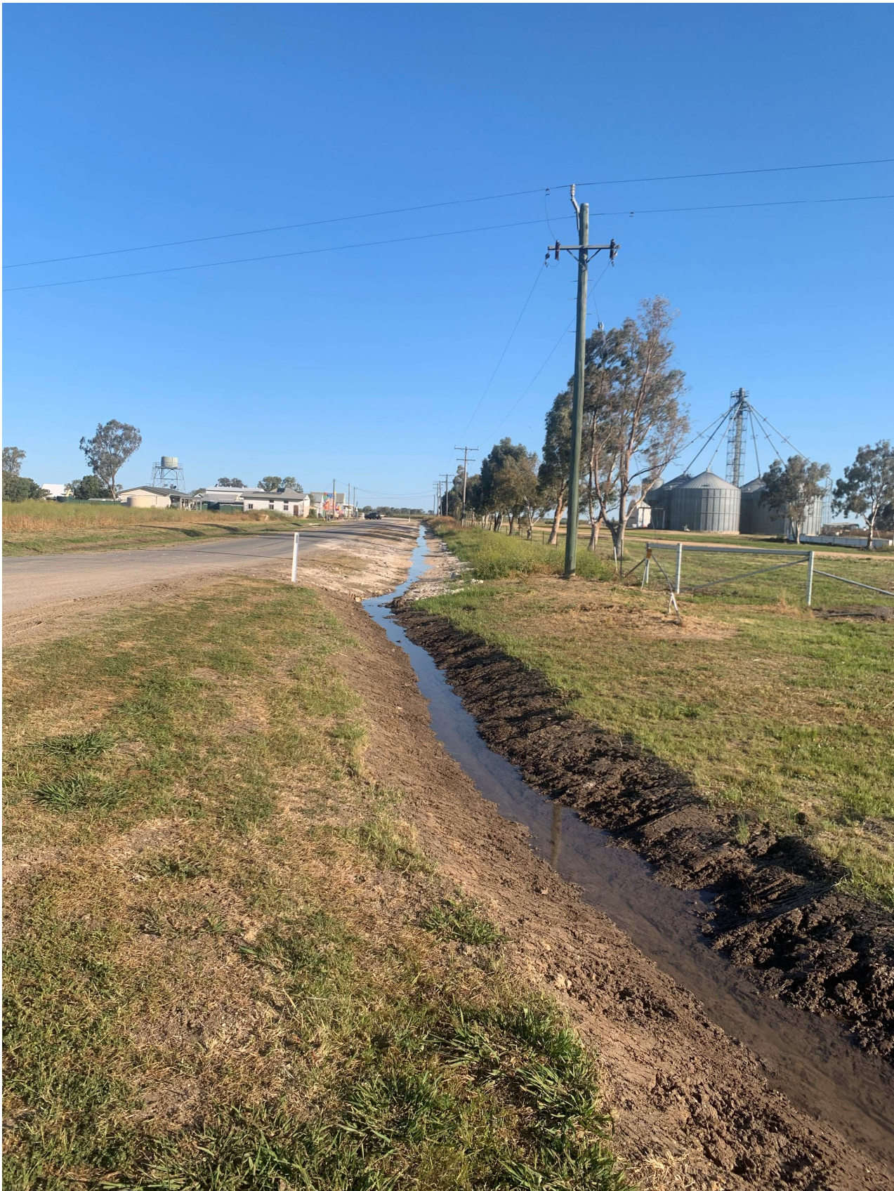
Figure 2 - After photo of same table drain from previous photo.
